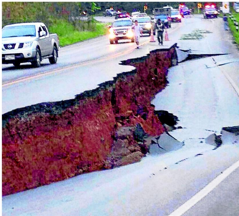
Motorists drive past a large crack in a highway caused by an earthquake in Chiang Rai province yesterday. EPA
